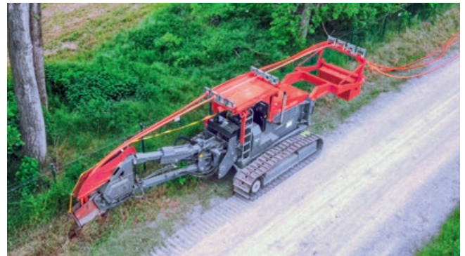
Individual cable guiding systems
