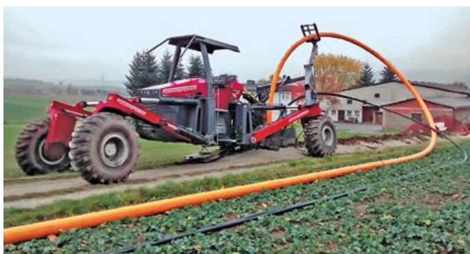
Plowing in of a gas pipeline PE-RC OD 180 and 2 x cable protection pipe OD 50
